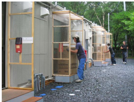
The delivery team is in a bustle, delivering and installing six electronic appliances sets in the prefabricated housing clusters in Ishinomaki, Miyagi. The electronic appliances continue to reach the surviving families across the nation. ©JRCS
